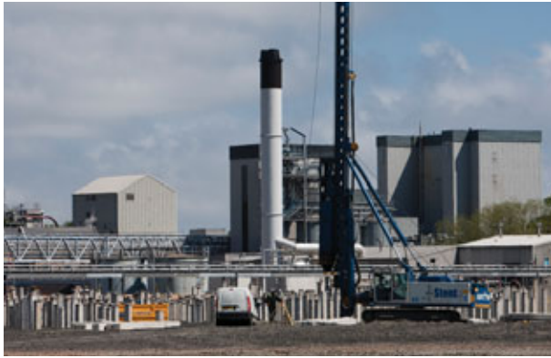
The new bioenergy plant at Cameronbridge is part of a development that will divert spent grain and wastewater to make the site largely self-sufficient in electricity
